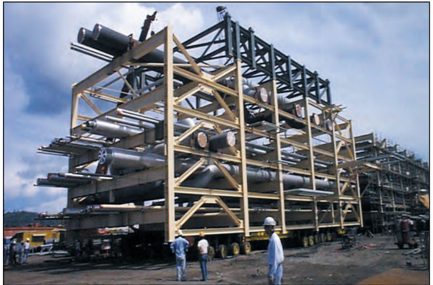
Plate 4.4 Typical pre-assembled pipe rack
