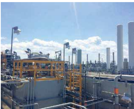
Plate 6.4 – Wastewater treatment plant at the LNG Plant site
