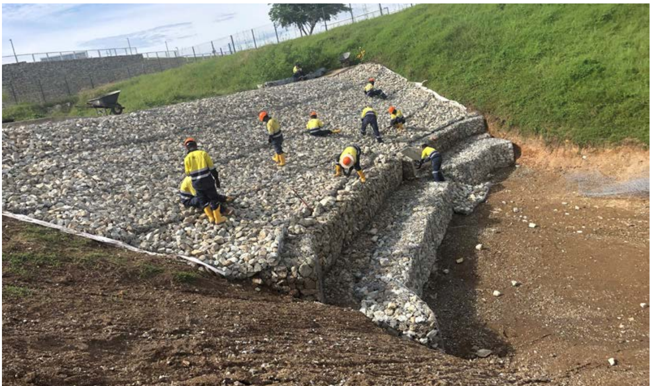
Workers tying gabion baskets on the ExxonMobil Haus stormwater detention pond during embankment repair
