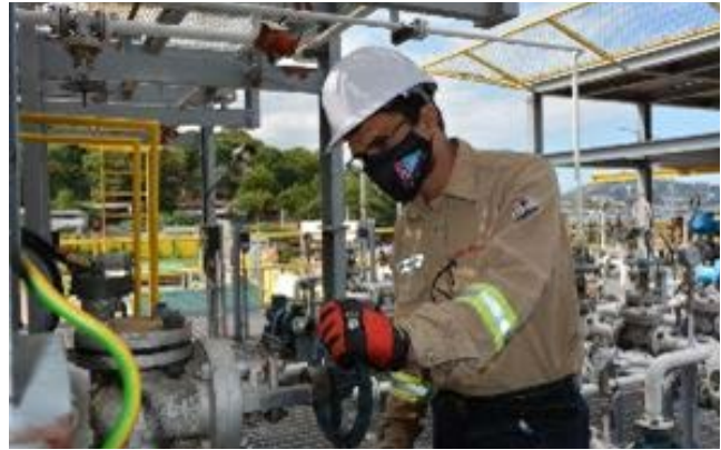
Integrity Engineer, Sebastian Hemetsberger, turns a main isolation valve at the Kumul Petroleum Academy safe live plant
