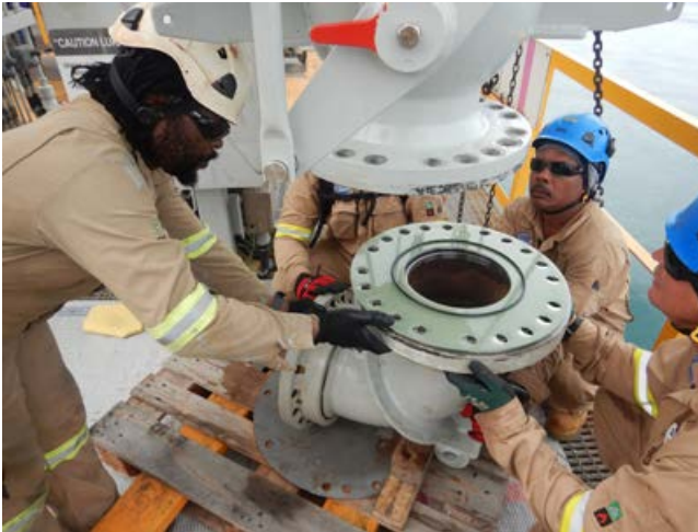
Newly recruited Technician Level 1 trainee, Tom Homoka (back right), learning how to install a new insulation joint at the LNG Plant Marine Terminal
