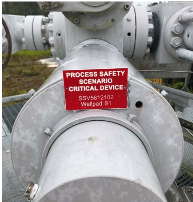
Signage installed at the HGCP indicating the device is part of critical safeguards for high consequence process safety scenarios
