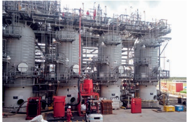
Train 1 dehydration bed molecular sieve unit at the LNG Plant
