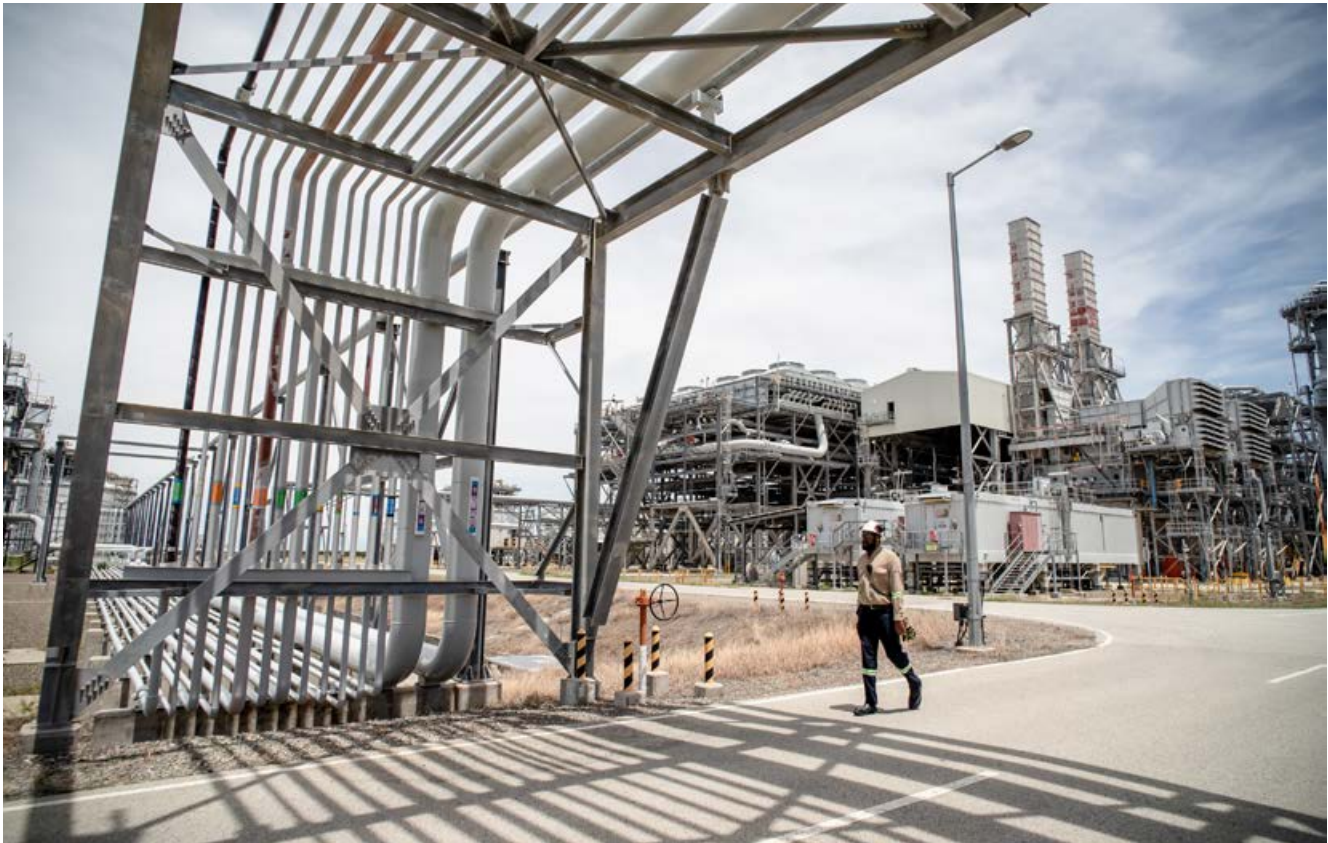
EMPNG Facilities and Process Surveillance Engineer, Elijah Lavai walking past a utilities pipe rack at the LNG Plant site
