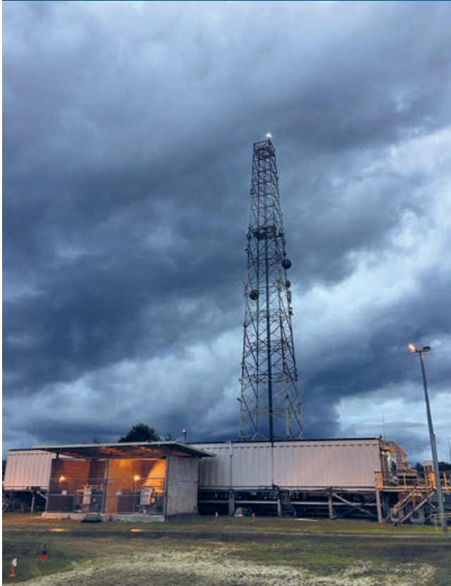
HGCP telecommunications tower
