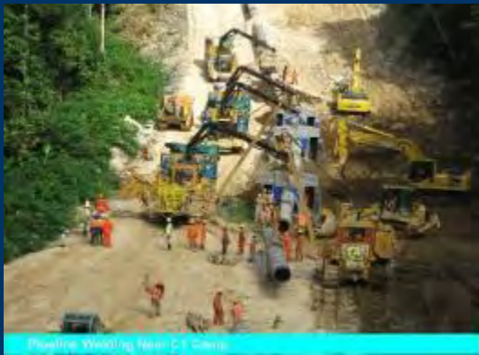
Reactive Working Near C.I. Sump
