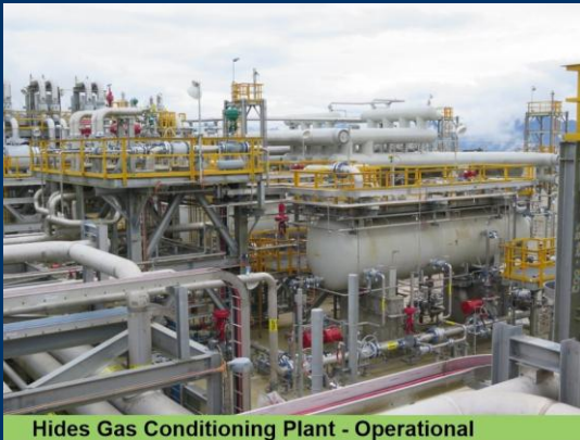
Hides Gas Conditioning Plant - Operational
