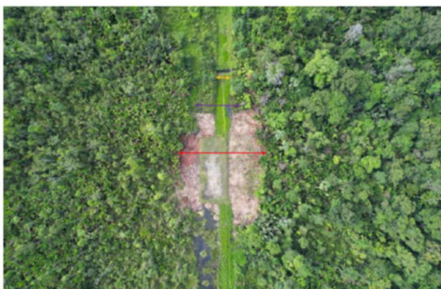
Helipad at KP290 with trees cut down to max width of 59m, beyond approved 30m construction allowance
