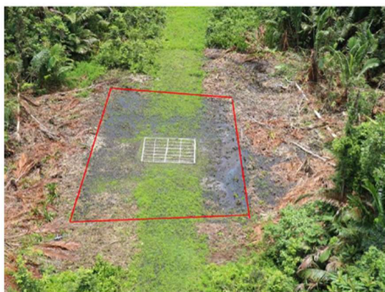
Helipad at KP284 with trees cut down to max width of 45m, beyond approved 30m construction allowance
